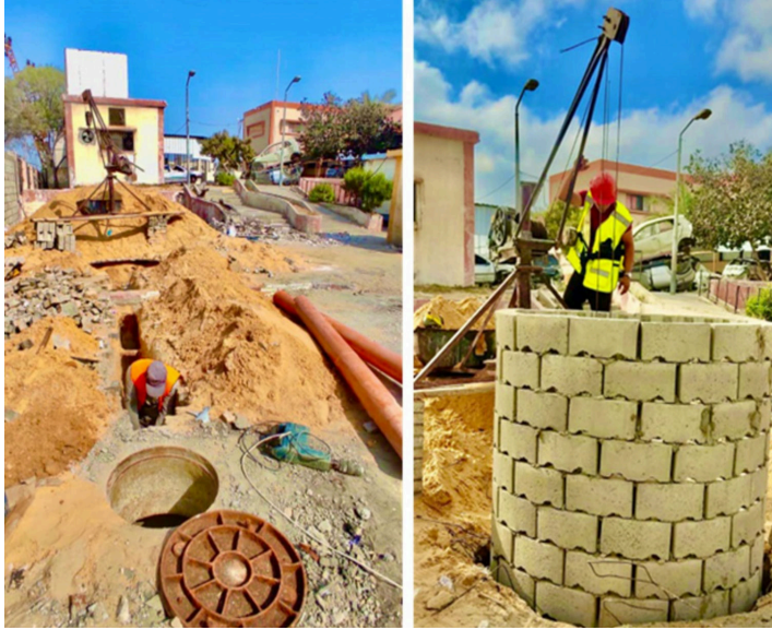
UNICEF supported the construction of four septic tanks at Nasser Hospital in Khan Younis to control sewage overflow.
